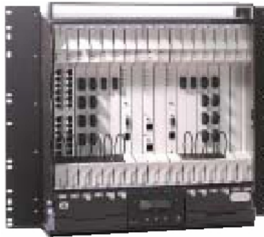
Figure 34: A CISCO Optical Transport Platform
